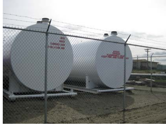
City of Hooper Bay ~ Bulk Fuel Tanks
